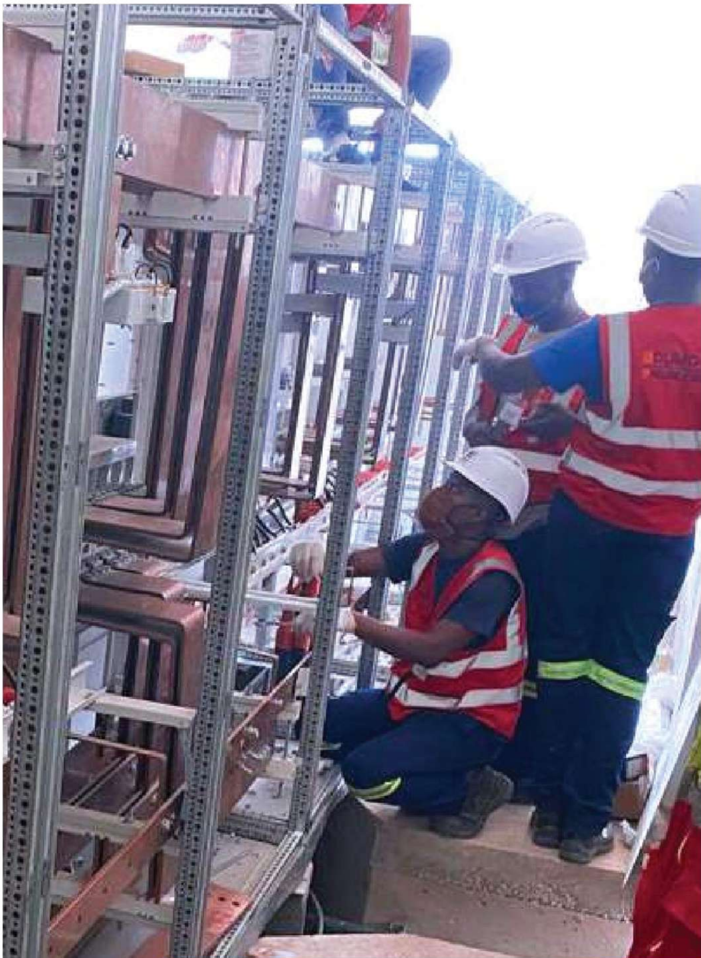
GHANA RUBBER, APIMENIM, LOW VOLTAGE SWITCHGEAR PANEL CONSTRUCTION
